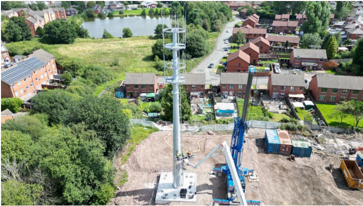
Figure 3 – Aerial imagery of a 30m-high tower deployed at Century Mill, George Street, Farnworth, BL4 9QW and approved by Bolton Council in 2022 (Source: Applicants drone imagery)
